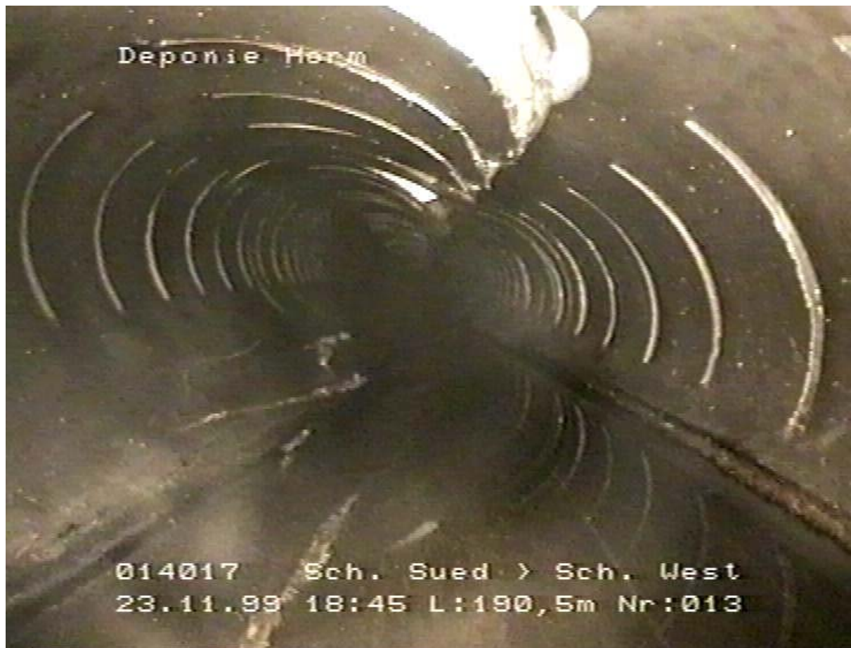
Figure 1: Damaged drainage pipe – axial crack
